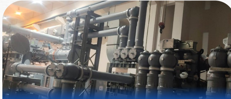
Expansion of GIS at Atul GETCO 220kV at Valsad (Government)
