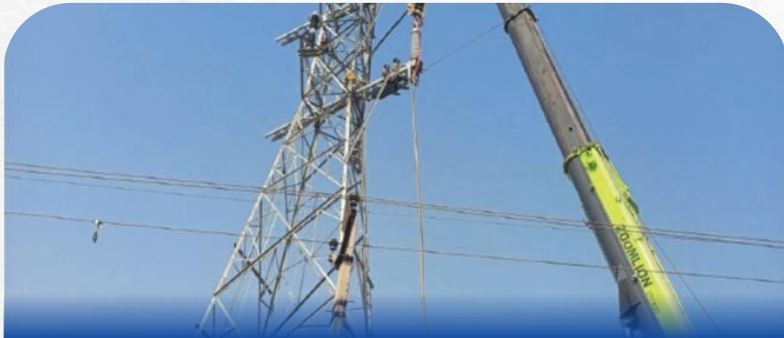
Lalgarh Traction Substation for Indian Railways, Bikaner (Government)
