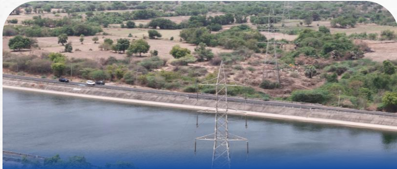
220 kV River Crossing Project (Government)
