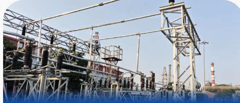
66 kV Substation – JK Paper Ltd. (Private)
