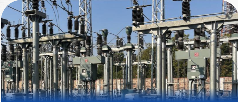
132 kV GIS Substation, TN-108 RVPN Project, Jodhpur (Government)
