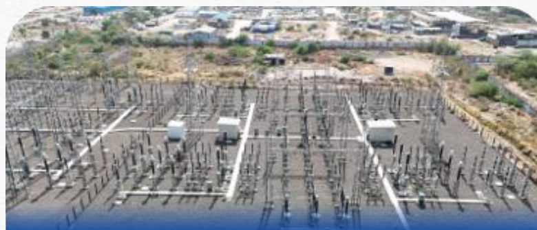
66 kV Power arrangement at GIDC Saykha (Private)
