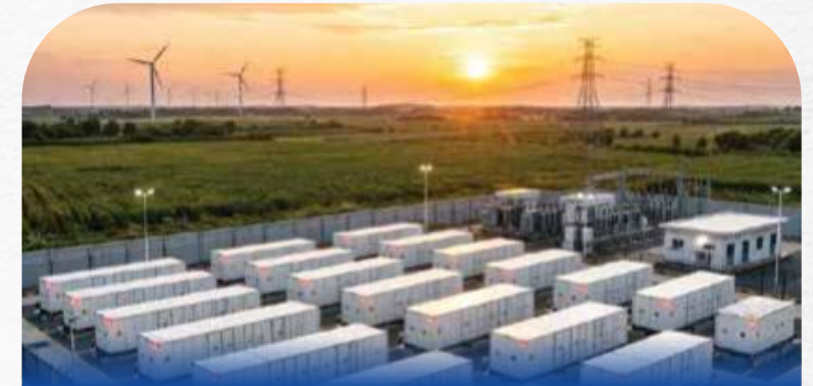
Battery Energy Storage System Project 65 MW / 130 MWh – Gujarat
