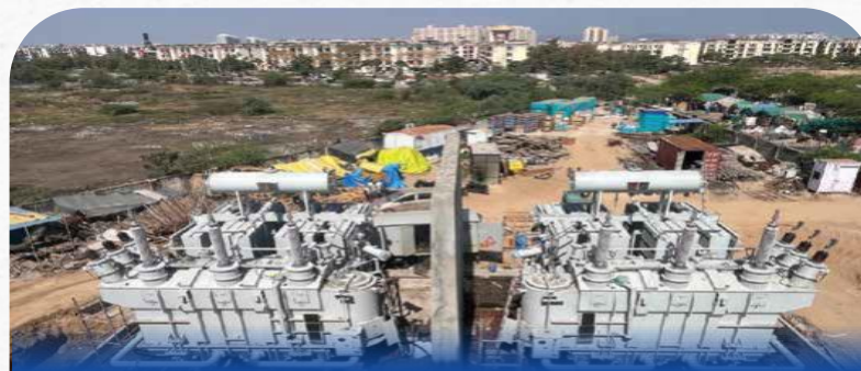
TN-119 Substation Project – Pratapnagar, Jaipur (Government)
