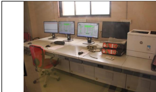
SCADA System Operations of EHV Substation
